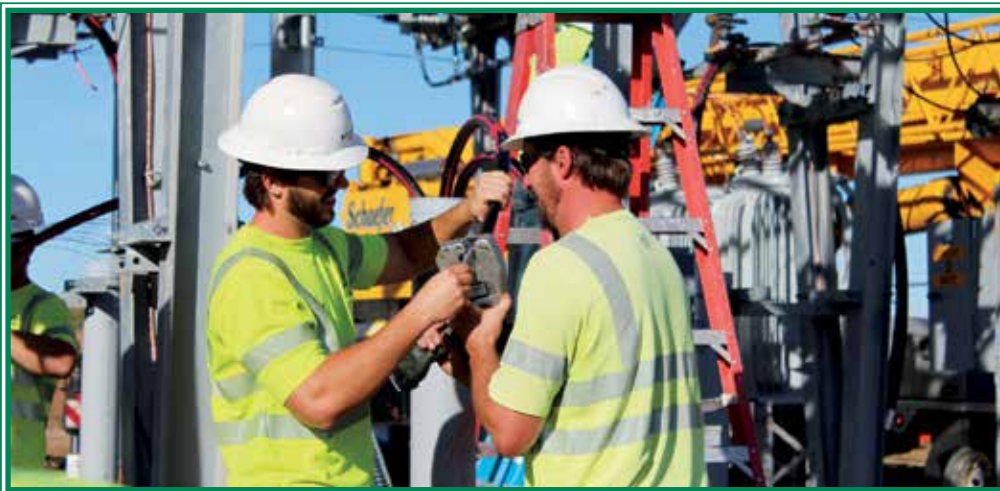
Linemen Tyler Moorman and Nick Neubert work together on the new Garden City Substation.
